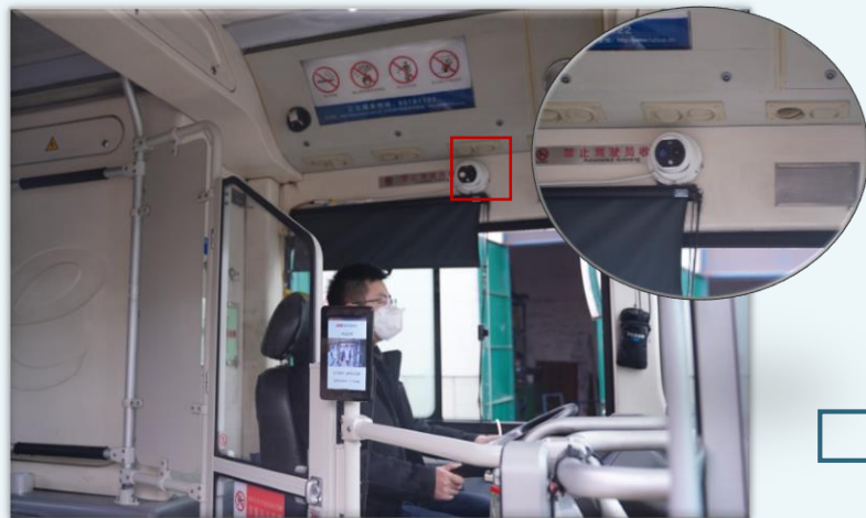
Camera installed at the top of the vehicle to face the entrance
