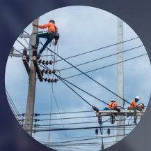
Electric power plant
