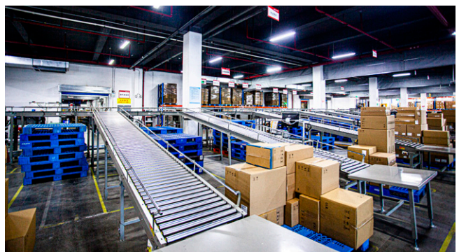
Automated Sorting Lines
