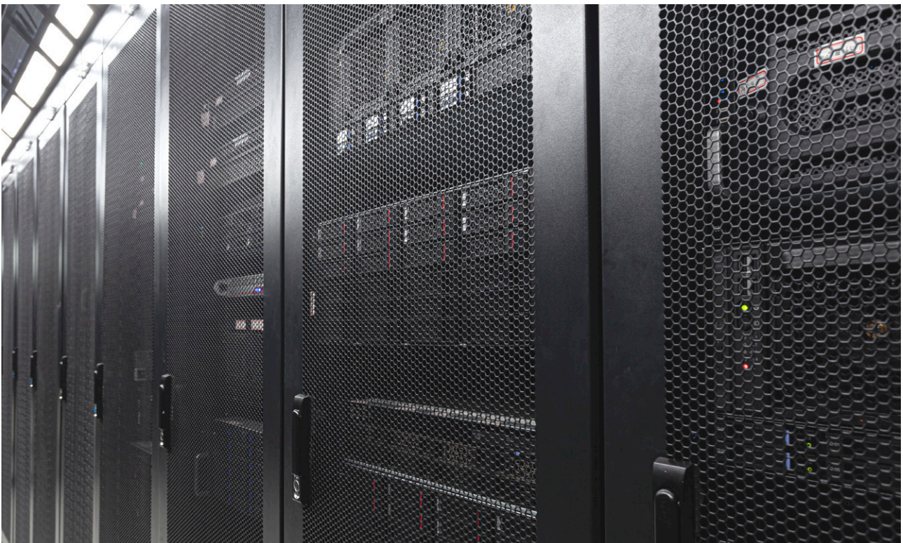
Verification Environment in G5 AI Cloud Lab Data Center
