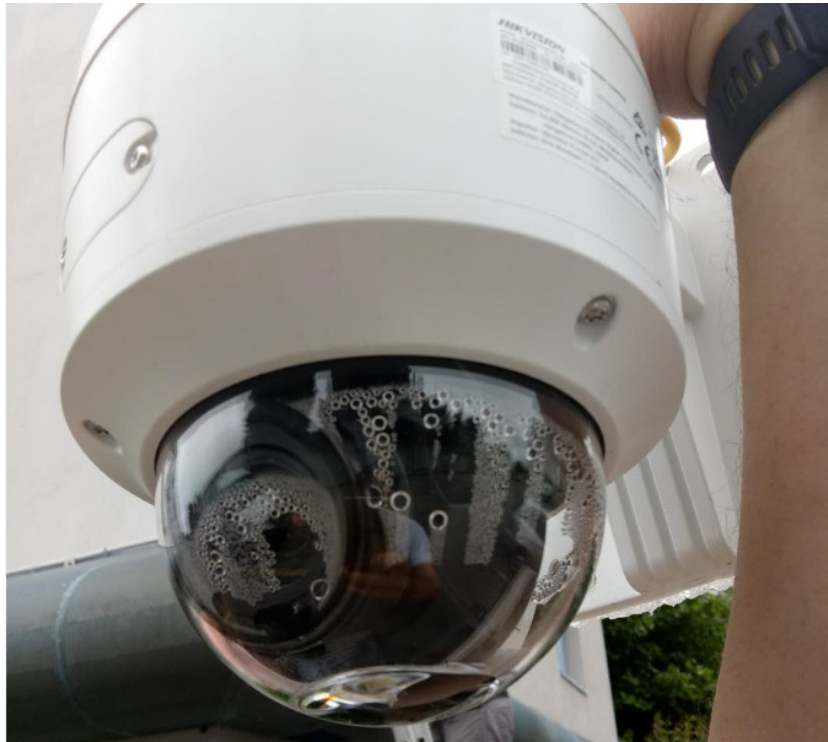
Figure 2, Water Ingress in Camera
